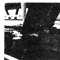
Fig.2 Defect of diagonal member in steel truss bridge.
