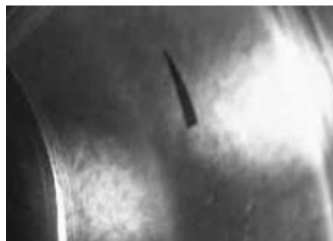
Fig.15 Inspection of a defect in piping.
