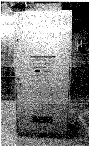
Fig.9 RCIC steam turbine controller
