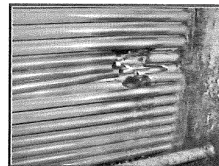
Fig.2 Damaged tube of main condenser
