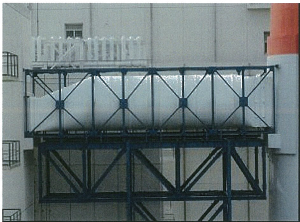
Phot.1 Main ducts
