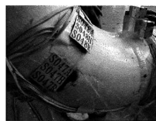
Fig. 8 Location of fatigue crack in Elbow1
