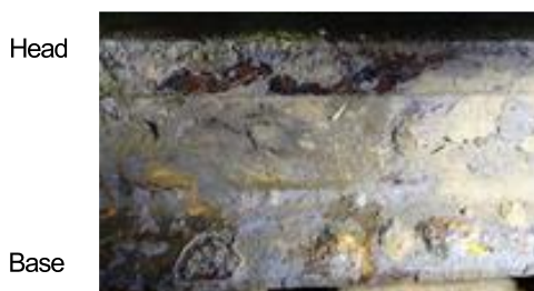
Fig. 1 Example of corroded rail (Side)
