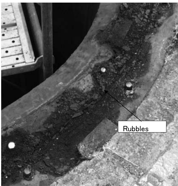
Fig. Photo of under base plate condition
