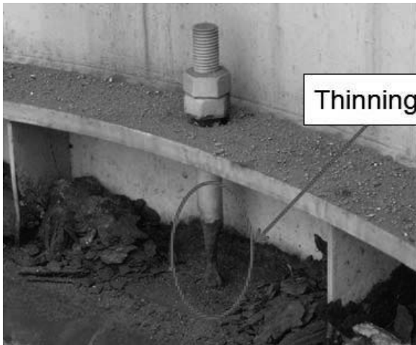
Fig. 4 Thinning of inner anchor bolt
