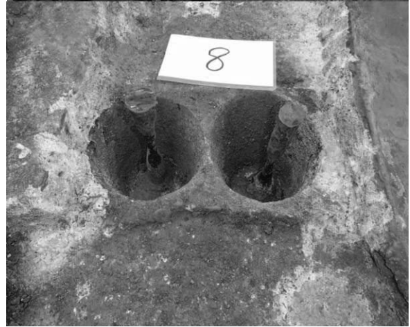
Fig. Thinning of anchor bolts in remain of wrapper tube
