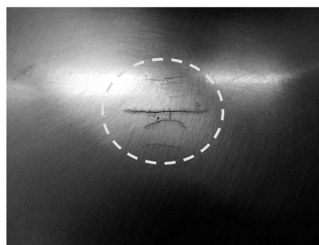
Fig.5 Example of the thermal fatigue crack
