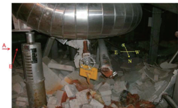
Fig.12 Photo of Moisture Separator after the earthquake
