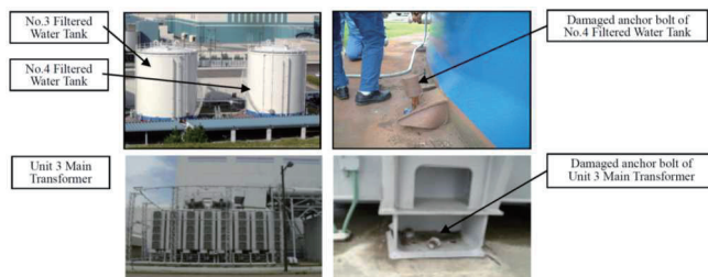
Fig.4 Anchor bolts fracturing of Filtered Water Tank and transformer
