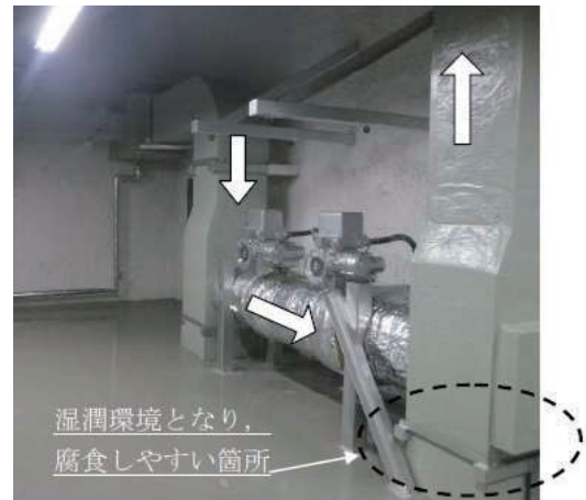
Fig.4 Low point of the air-conditioning duct
