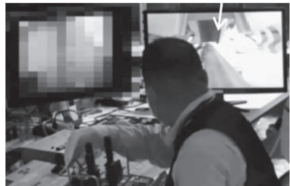
(3)Remote control room
