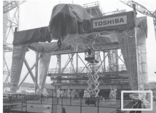
(1)View of the fuel handling equipment
