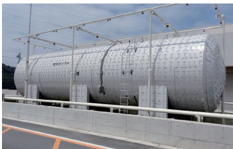
Fig. 7 Shock absorber mounting condition on heavy oil tank
