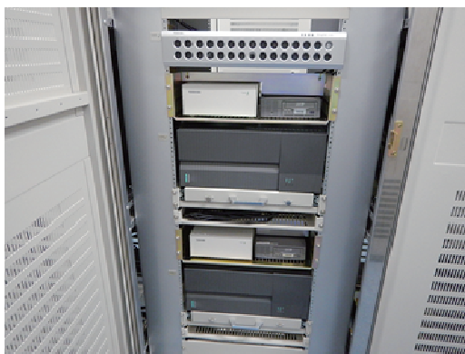
Fig.4 : Equipment taken out to the factory (before updating)
