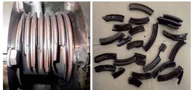
Fig.1 The broken exhaust pipe expansion joint & fragments of the broken bellows
